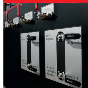
Three-way control of the liquid
