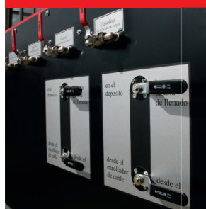
Three-way control of the liquid
